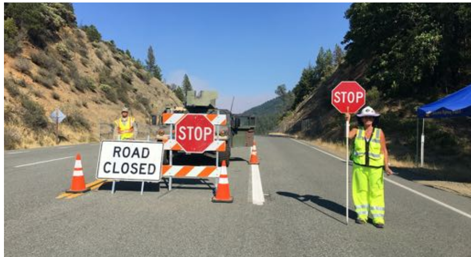
Road closure east of Weaverville in Trinity County.
